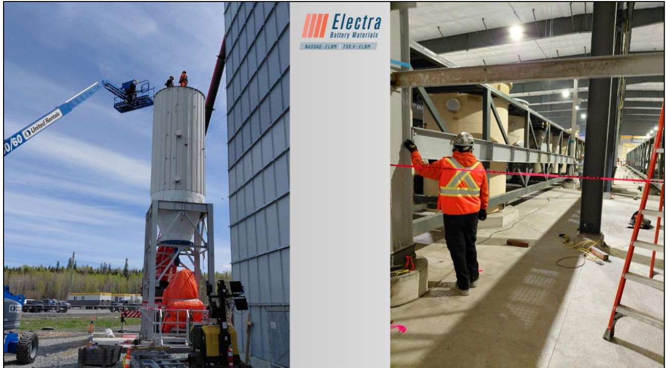
Images above: Construction progress at Electra's refinery. Left: Contractors erecting the cobalt sulfate storage silo. Right: Contractors installing structural steel for the solvent extraction plant internal pipe rack.
